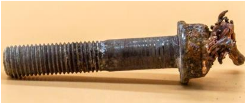
Figure 2 - A bolt that had rubbed through a power cable with the copper cable still welded to the head.
